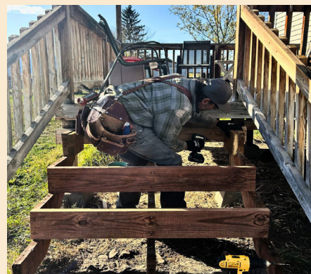
Peter Bushman worked with MAS to repair wooden steps for a client.
